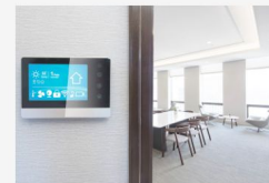
Real-World Applications of Commercial Lighting Control Systems
